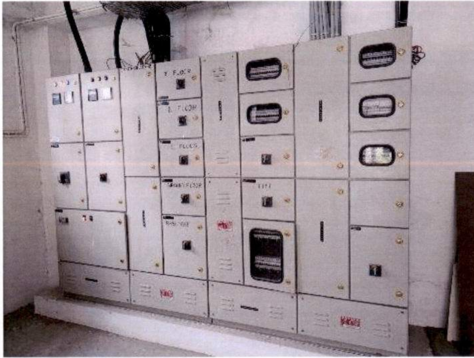
Figure 5-3: Main PCC panel in panel room of science block
