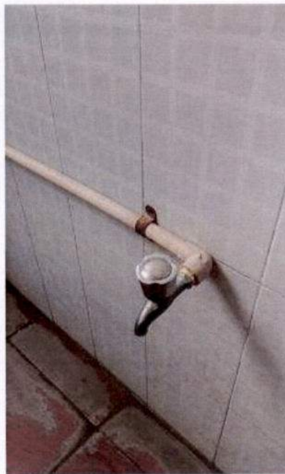
Figure 4-25: Sample photo of hot water tap in boy's hostel
