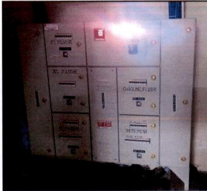
Figure 5-9: Electrical distribution panel – Girl’s hostel (new block)
