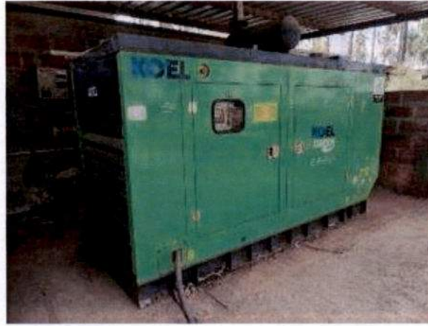
Figure 5-15: Diesel Generator (DG) set – Girl's Hostel
