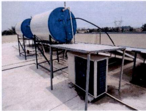
Figure 4-23: Solar water heater with Heat pump system – Women’s hostel
