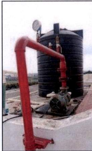
Figure 4-8: Connection for fire hydrant system – Management block
