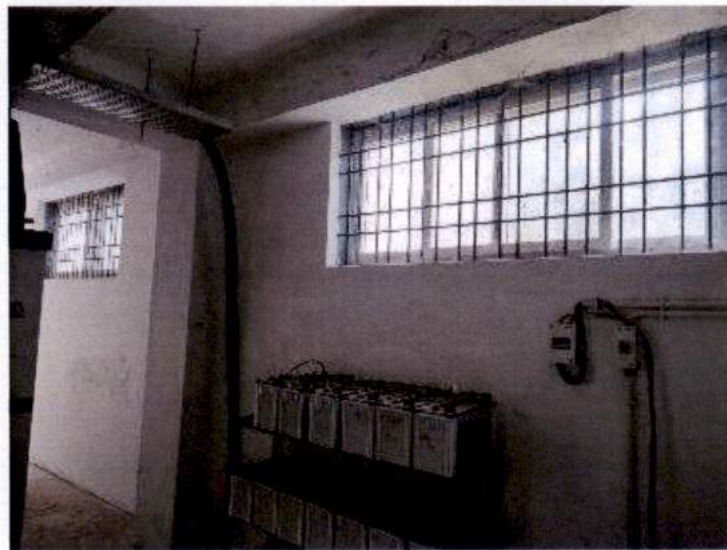
Figure 5-23: Well-ventilated and day-light integrated Panel room
