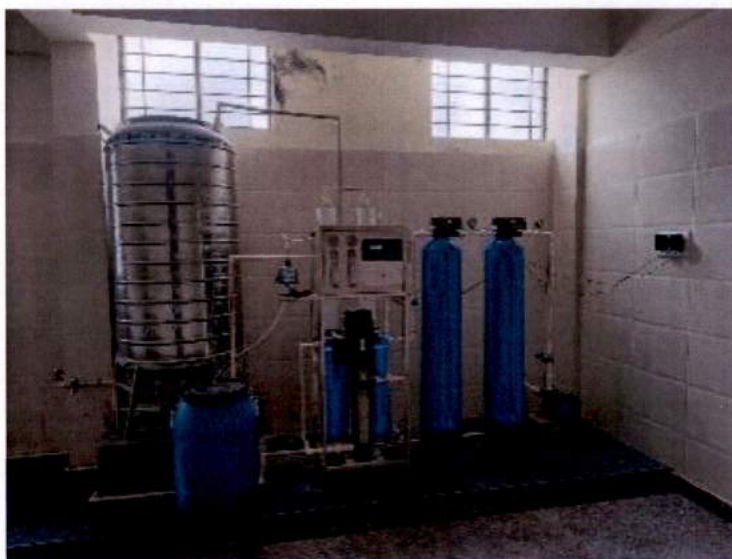
The RO plant (500 lph) installed at women's hostel new block
