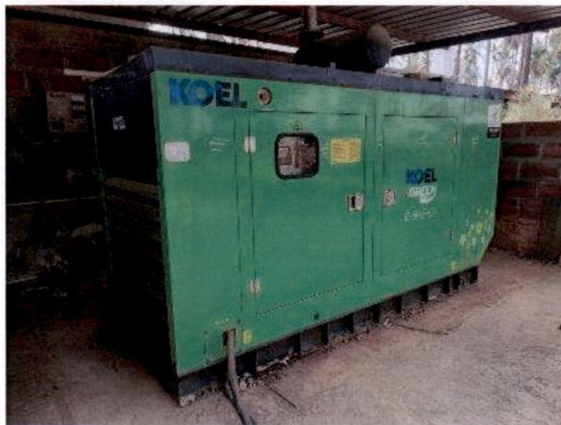
Figure 5-14: Diesel Generator (DG) set – Boy's Hostel
