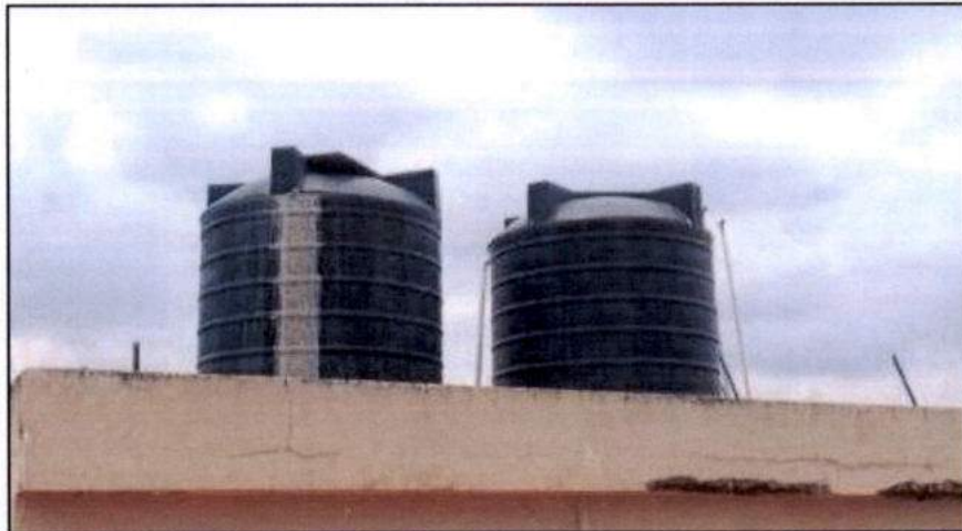
Figure 4-11: PVC OHT's – New Boy's Hostel – 2 (Amogha – Left wing side)
