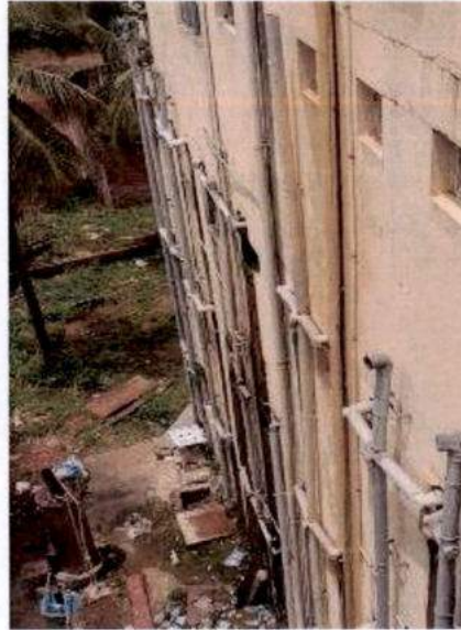
Figure 6-3: Waste Water Outlet Pipes
