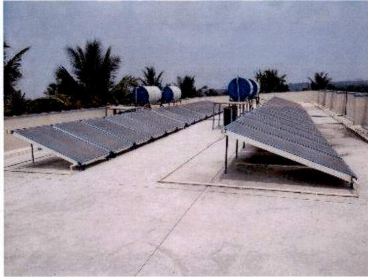
Figure 5-28: Women's hostel – Solar Water Heater system
