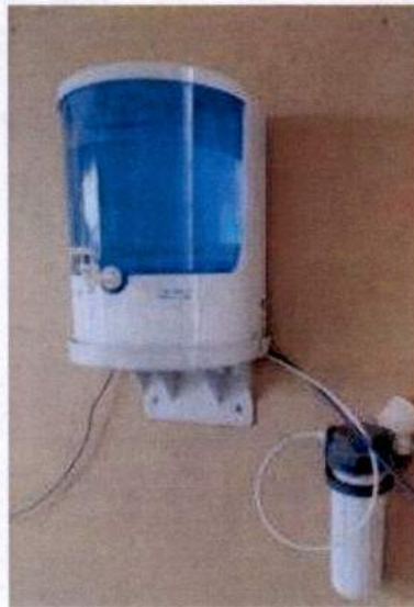
Figure 4-20: RO filter – Management block
