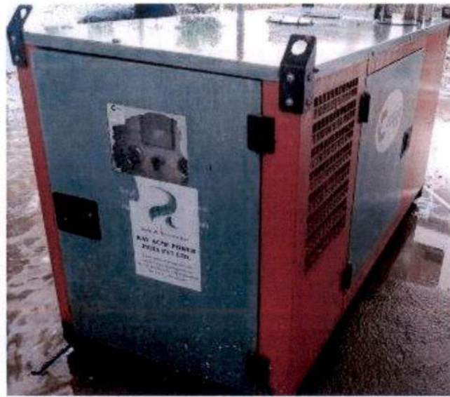
Figure 5-13: Diesel Generator (DG) set – Management Block
