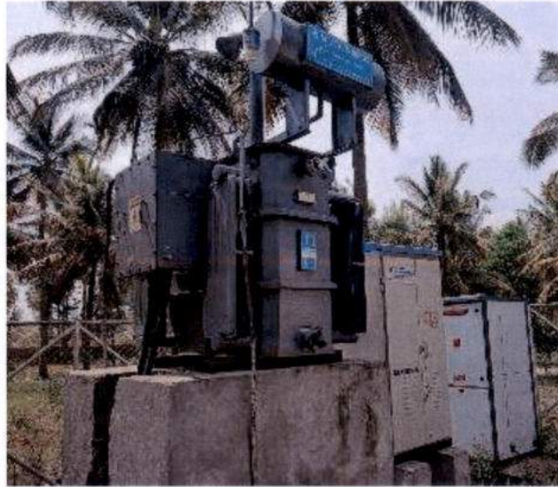
Figure 5-2: Hostel - Transformer yard
