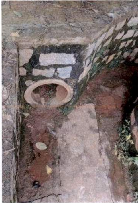
Figure 4-34: Dedicated rain water pipeline for pond
