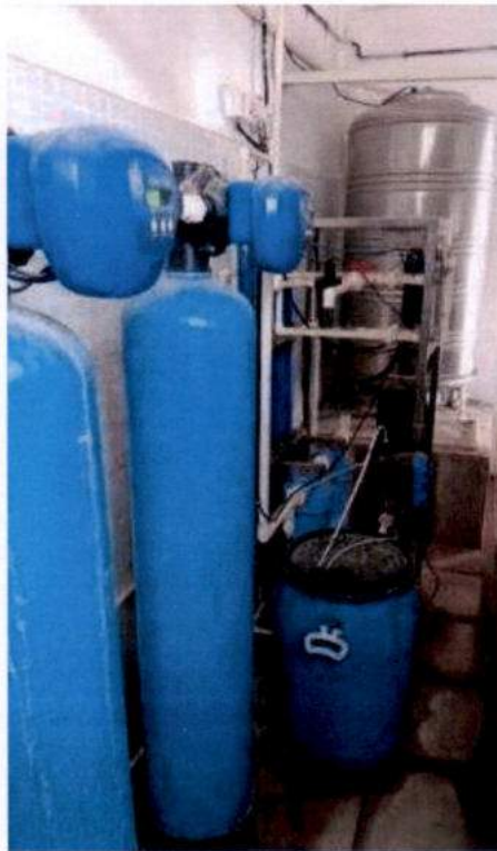
Figure 4-15: RO water treatment plant in boy's hostel
