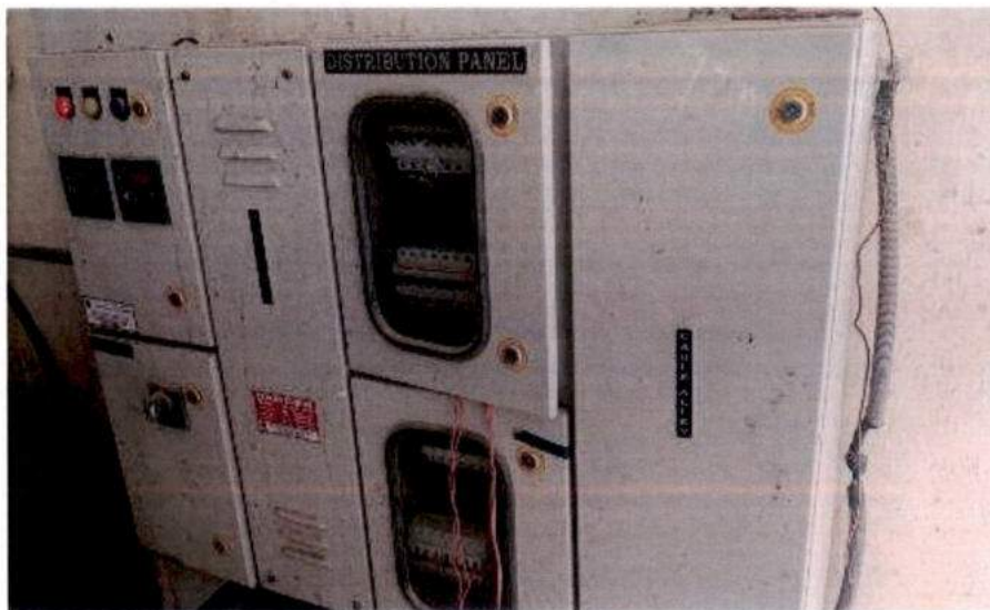
Figure 5-7: Electrical distribution panel – Boy's Hostel – 2 (Amogha block)
