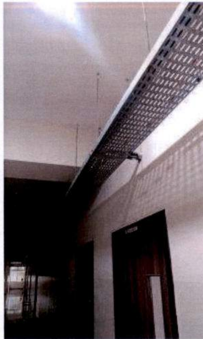
Figure 5-34: Cable Tray – Science Block
