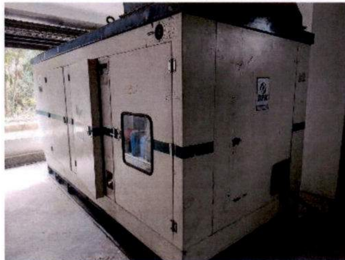
Figure 5-12: Diesel Generator (DG) set - Science block
