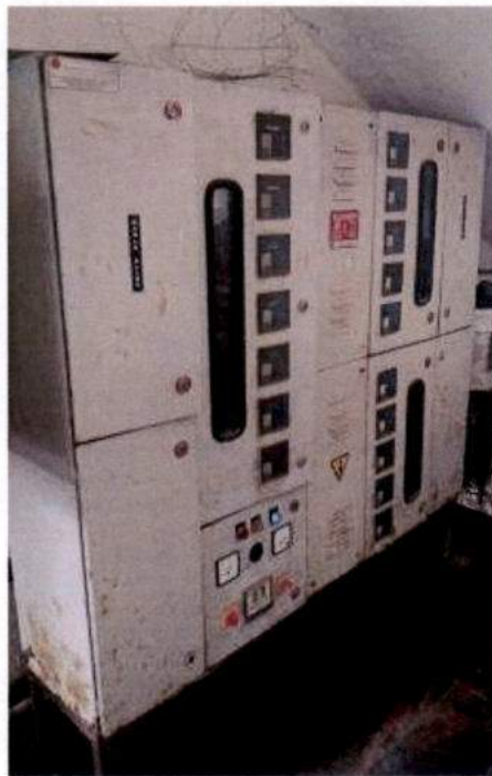
Figure 5-6: Electrical distribution panel – Boy's Hostel
