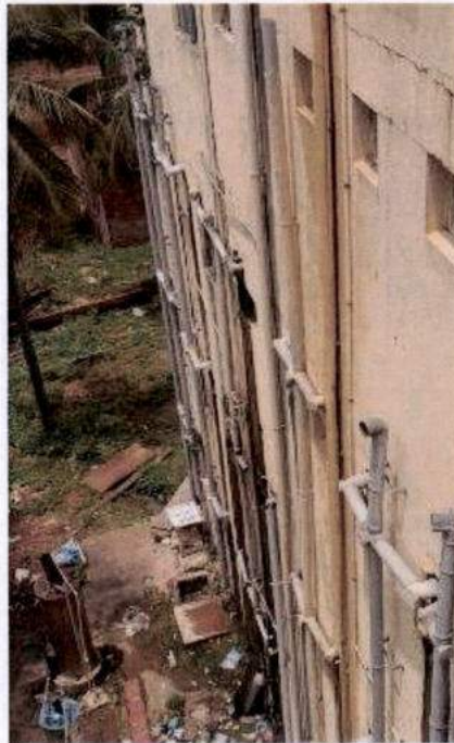
Figure 4-28: Waste Water Outlet Pipes
