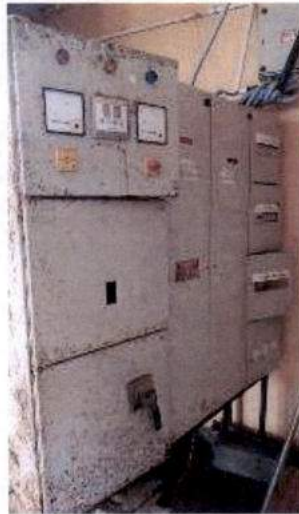
Figure 5-4: Electrical distribution panel – Management block
