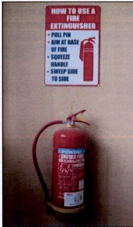
Figure 3-2: Fire Extinguisher with instructions to use
