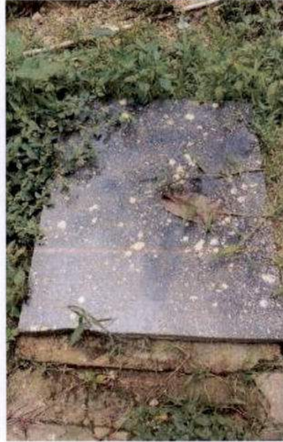
Figure 4-29: Waste Water Chamber
