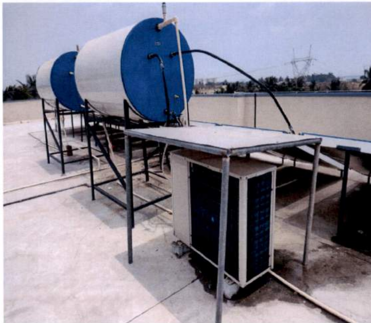
Solar Facility in the campus
