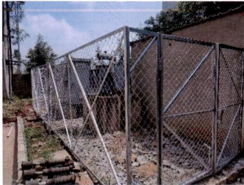
Figure 5-1: Transformer Yard - College
