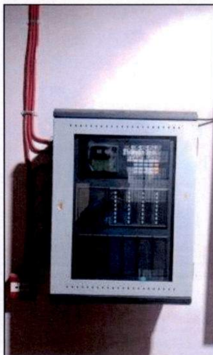
Figure 3-3: Fire Alarm Control Panel
