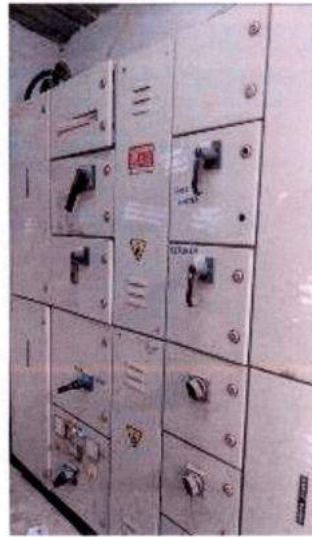
Figure 5-5: Main LT Electrical Distribution Panel – Boy's Hostel
