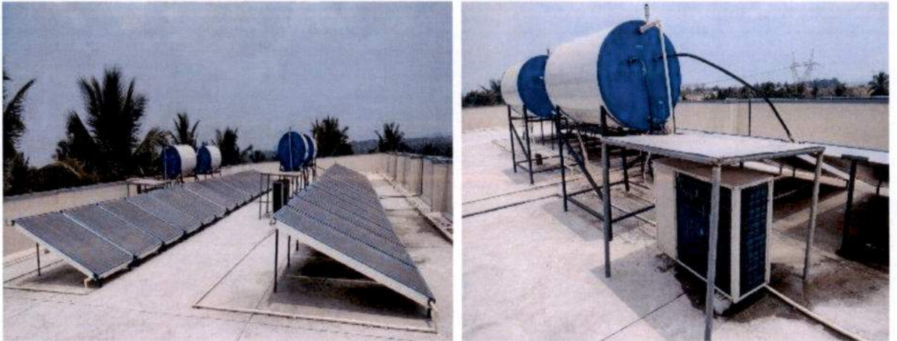
Figure 4-39: Use of Solar Water Heater
